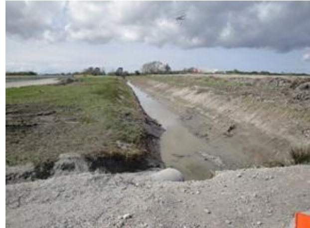
Drainage leading to 72 nd Street
